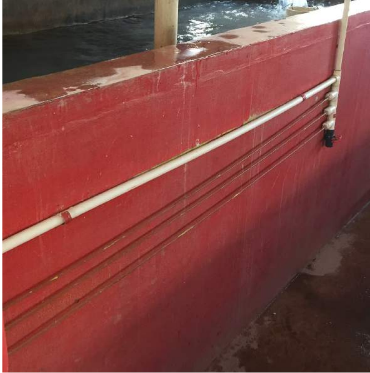
Figure 1: CDC manifold system to which these governing equations refer to. Image taken at an AguaClara plant in Honduras.
