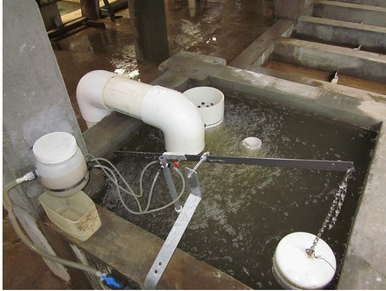
Figure 9: Current (as of July 2011) LCDC installed at the Marcala El Chiflador 2 AguaClara plant
