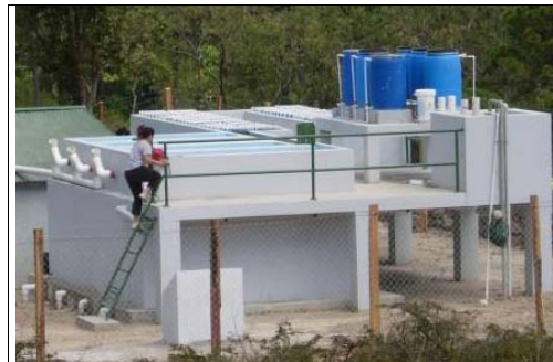
Figure 3. AguaClara water treatment plant in Ojojona Honduras.
