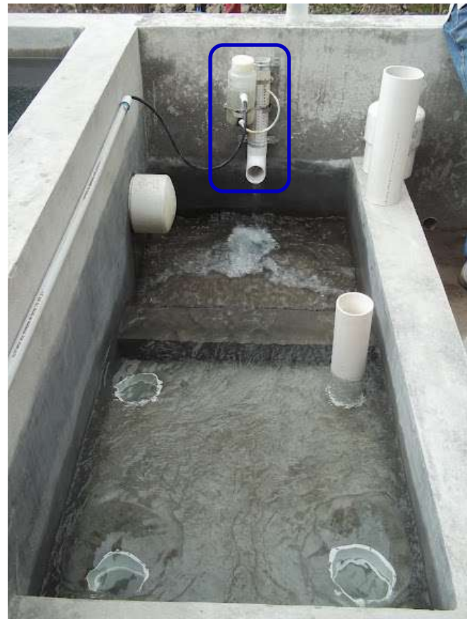
Outlet Box – Filtered water leaving for distribution tank
