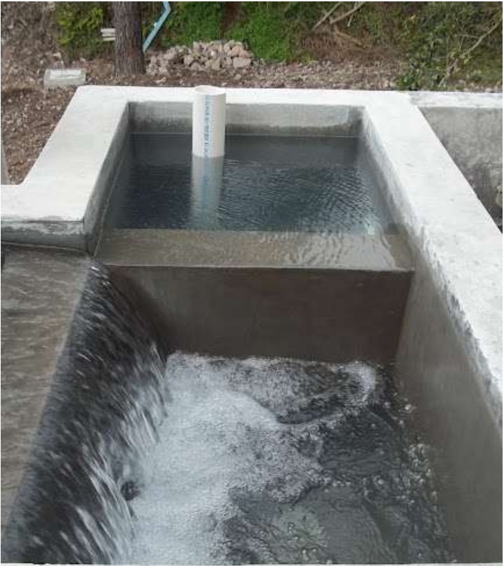
Inlet Box - Water arriving from sedimentation tanks
