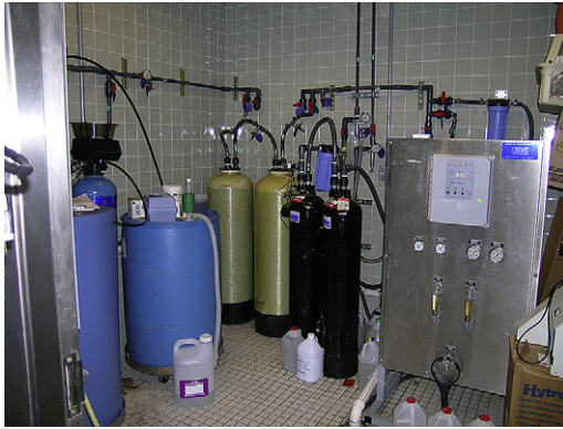
Fig. 4. Example of a water treatment system.
