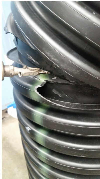
Figure 5: The thin walls of the pipe make welding a delicate process. Too much heat or pressure can lead to a puncture in the tank.
