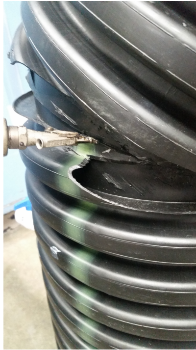
Figure 4: The thin walls of the pipe make welding a delicate process. Too much heat or pressure can lead to a puncture in the tank.
