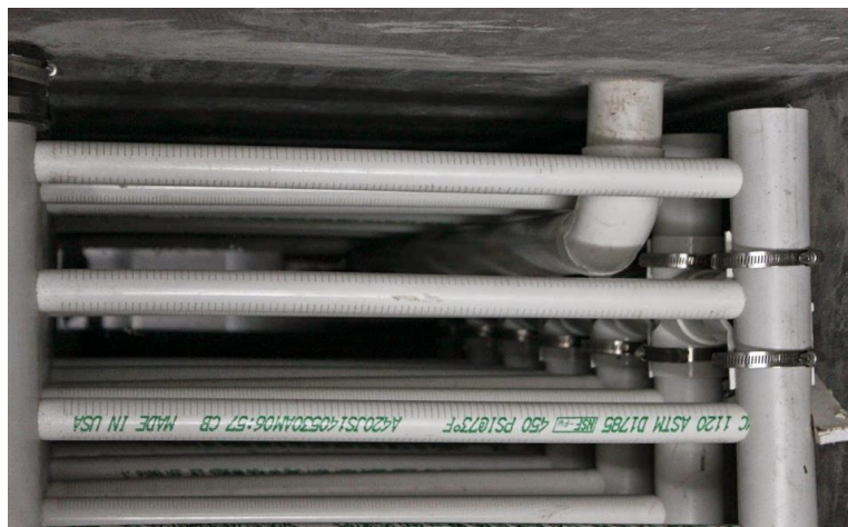
Figure 1: Slotted Pipes are currently used for sand filter. The slots shown in this figure are prone to be clogged with sludge and other particles.
