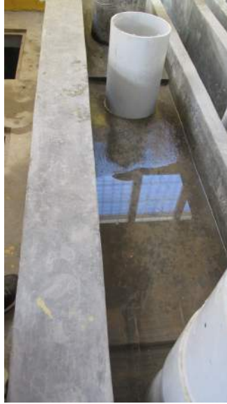
Figure 1: Sedimentation Tank Inflow Weir (San Nicholas)
