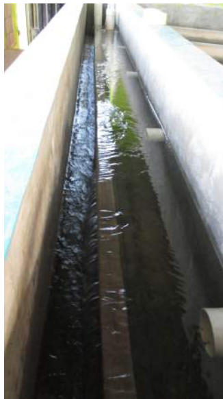
Figure 2: Sedimentation Tank Effluent Launder (Atima)
