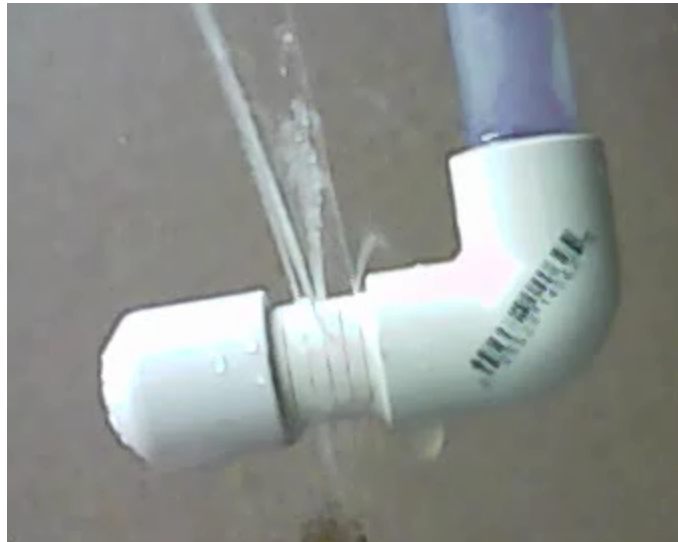
Figure 5: Clean Water through Clogged Slotted Pipe Immediately after Experiment
