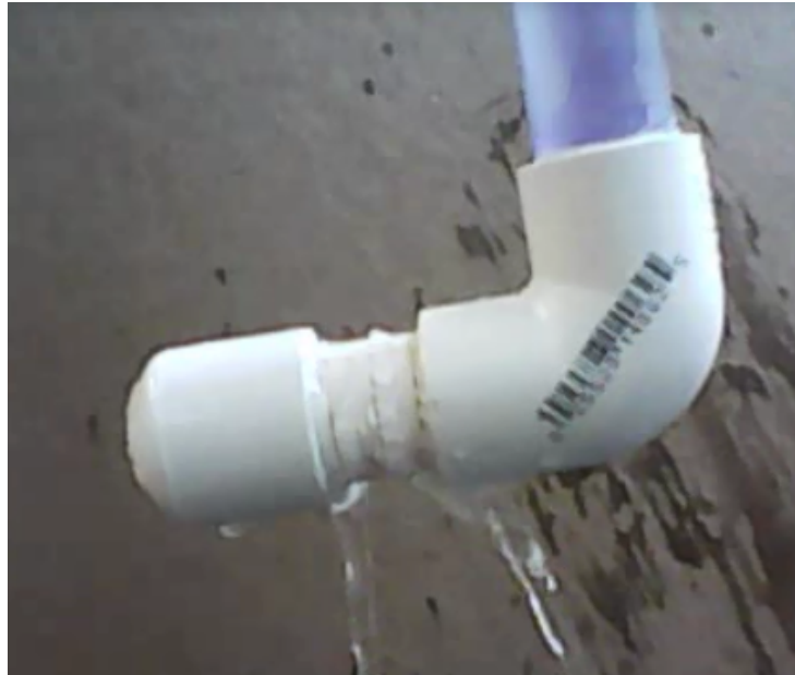
Figure 6: Clean Water through Clean Slotted Pipe
