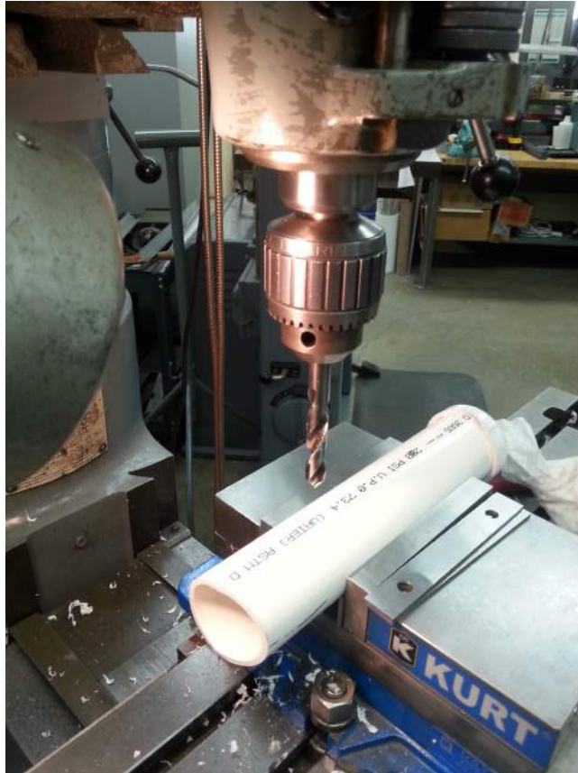
Figure 11: Drilling the manifolds According to the process described in 10, the manifolds were milled to allow for the insertion of slotted branches. The slotted branches themselves were also milled in this way later in the construction process.
