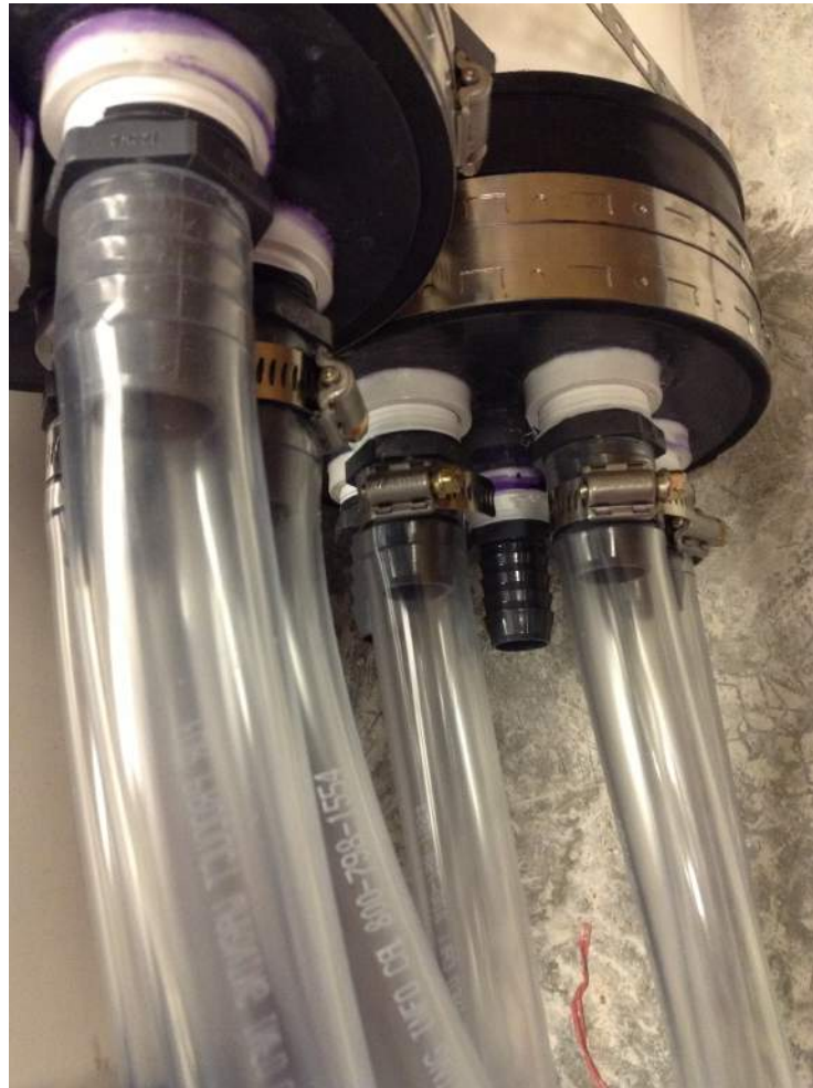
Figure 15: Flexible tubing and hose clamps, both of 2.54 cm diameter, were used to connect the inlet and exit tanks to the side of the main filter column.
