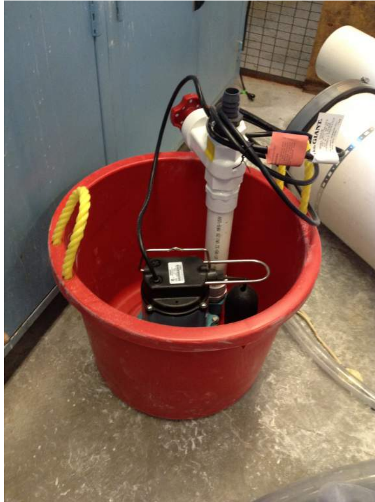
Figure 27: Recycling Pump The Little Giant Pump that recycles water through the filter. This pump is set to provide a flow rate of 0.8 L/s and pumps directly into the filter’s entrance tank.
