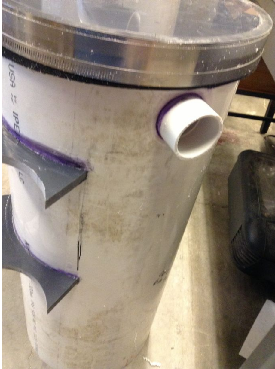
Figure 17: Backwash Pipe Construction This 3.81 cm coupling, which will ultimately fit the backwash pipe, was glued into the side of the filter column, close to the top cap. This hole was drilled with a 5.72 cm hole saw whose blades had been sanded slightly inward. The coupling was attached with PVC glue.
