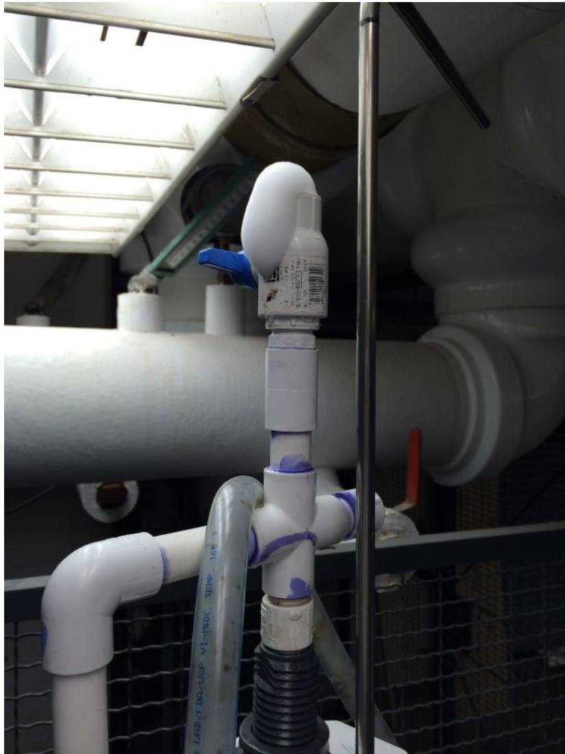
Figure 4: Bubble Test Result The valve at the top of the column after the bubble test showing a significant air leak.
