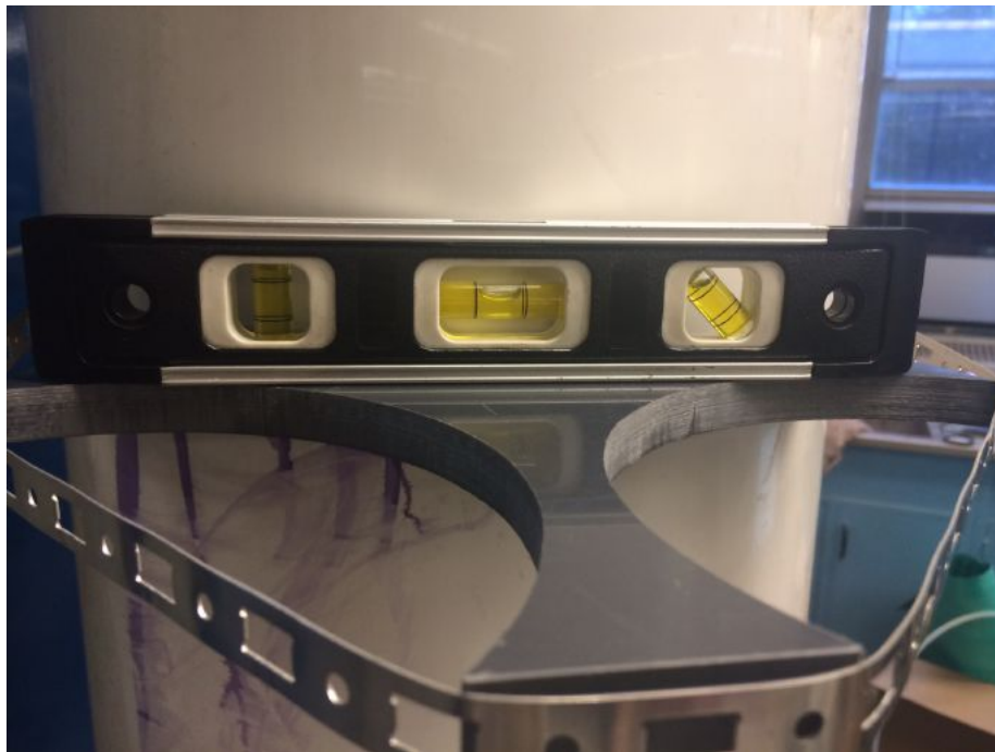
Figure 15: Attaching Spacers with Level The two spacers were attached to the side of the filter column using PVC primer and PVC glue. They were placed so as to be parallel with the floor; this was ensured with the use of a level. Once glued, they were secured to dry with a hose clamp.
