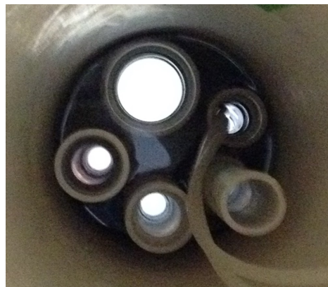
Figure 5: The four entrances to the tubes that enter the filter column (the pipe that corresponds to the bottom-most inlet tube is the pipe with the largest diameter)
