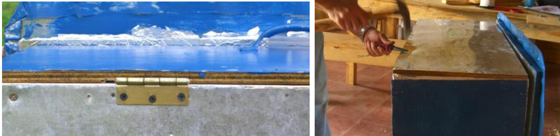
Figure 4: Left- Screw in the hinges on the bottom side of the cooker. Right- Attach the sheet metal to the front of the door using 1/4" or 1/2" screws or nails
