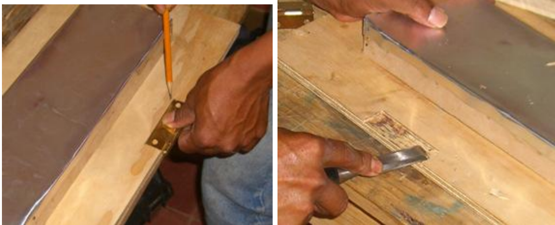
Figure 3: Left- Trace the door hinge in place. Right- use a chisel to cut out a recessed area for the door hinge.
