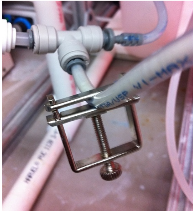
Figure 7: Clamp added to Floc Recycle Line
