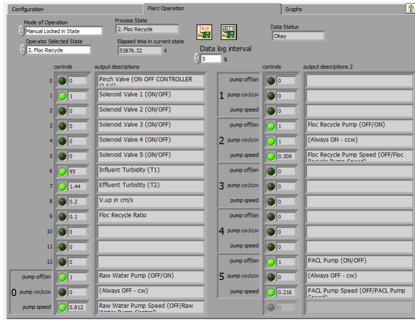
Figure 9: Process Controller Plant Operations
