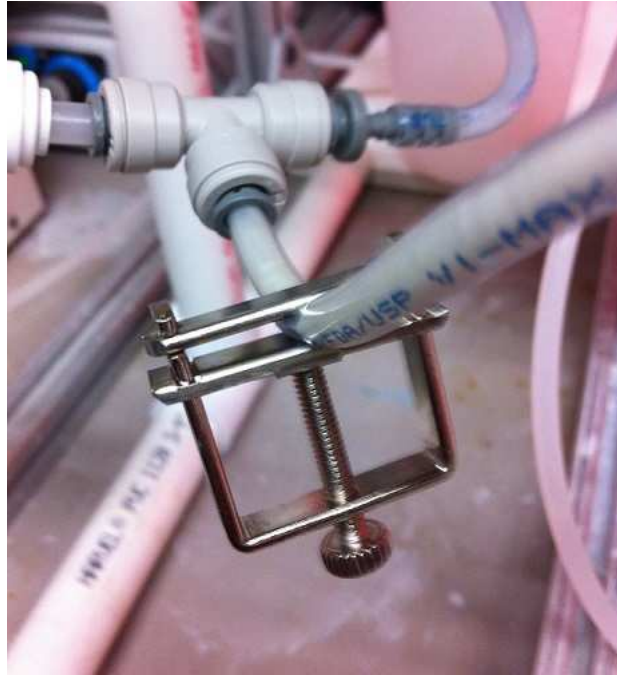
Figure 7: Clamp added to Floc Recycle Line
