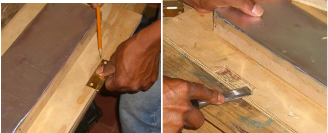
Figure 1: Left- Trace the door hinge in place. Right- use a chisel to cut out a recessed area for the door hinge.
