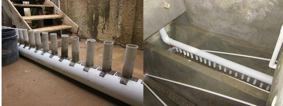
Figure 1: Spring 2011 version of the sedimentation tank inlet manifold and diffusers. These diffusers do not provide the continuous line source that is required to suspend all flocs that slide down the slopes of the sedimentation tank. In addition, the flat sludge drain cover does not provide the geometry for a jet reverser that can easily suspend the settled flocs.
