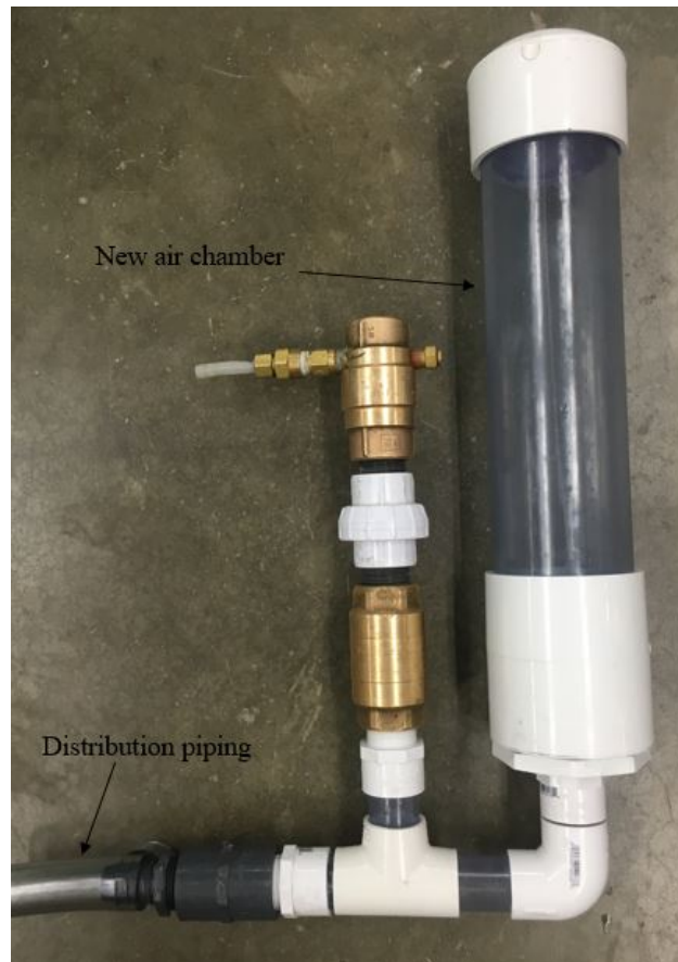
Figure 26: A second air chamber was installed next to the ram pump exit and behind the distribution piping in order to eliminate the vacuum effect.
