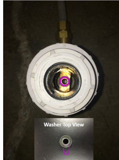
(b) A washer was added between the check valve and the problematic collar, to prevent the pump from jamming. Note that the diameter of the washer's opening is smaller than that of the collar, to effectively screen the edge of the collar from the check valve.
