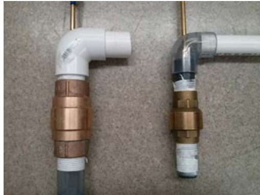
Figure 7: Waste valves - 1 inch (L) and \frac{3}{4} inch (R).
