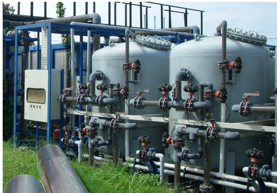
Abandoned package plant in La Ceiba, Honduras
