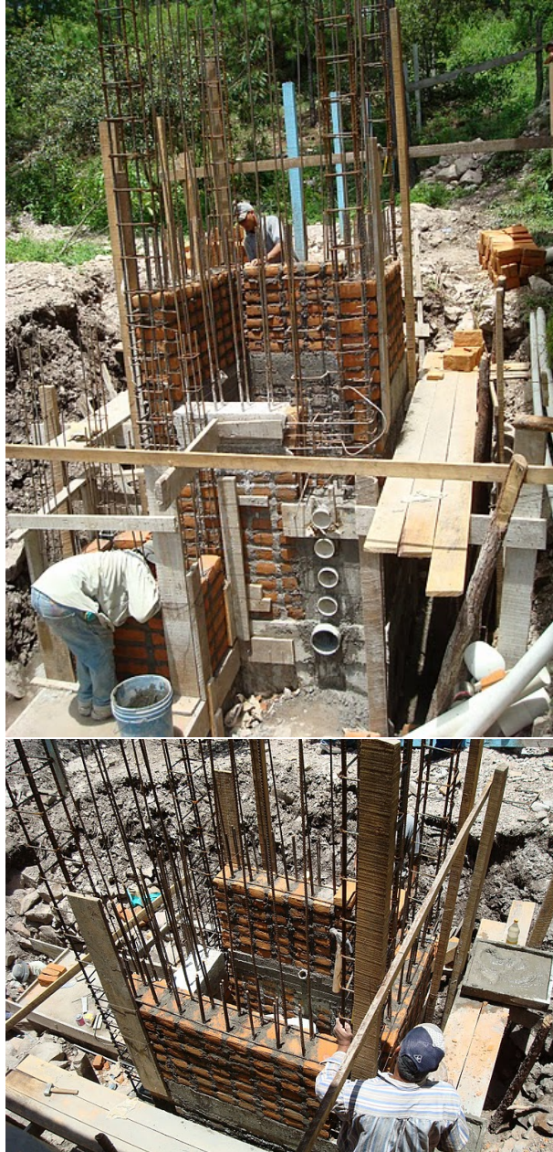
Figure 3: Re-bar and brick placement for the first stacked rapid sand filter at Tamara, Honduras. The concrete ledger is also visible.
