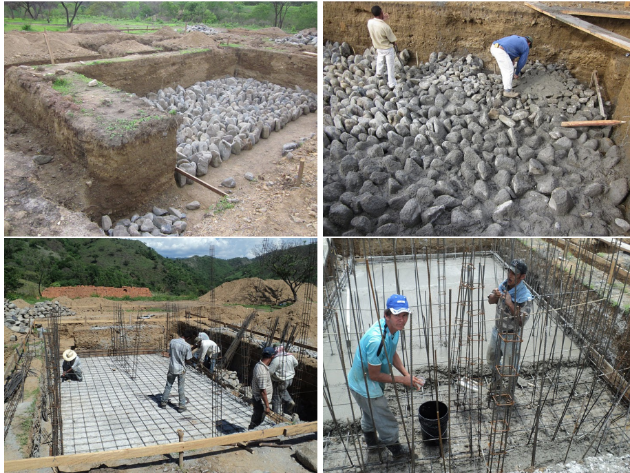
Figure 1: Construction technique for the slab at a 12 L/s plant at Alauca, El Paraiso, Honduras during the summer of 2011. The section of the slab with few vertical re-bars will support the sedimentation tanks. The vertical re-bars will support the channel walls for the flocculator.
