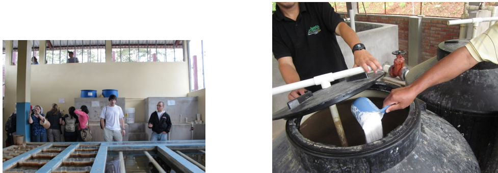
Figure 1: Coagulant stock tanks (blue drums in middle of the photo on the left) provide more than 24 hours supply of liquid coagulant. The chlorine tanks (photo on the right) contain a concentrated bleach solution made from calcium hypochlorite. The pipe mixing device used to stir the chlorine solution is visible on the right.
