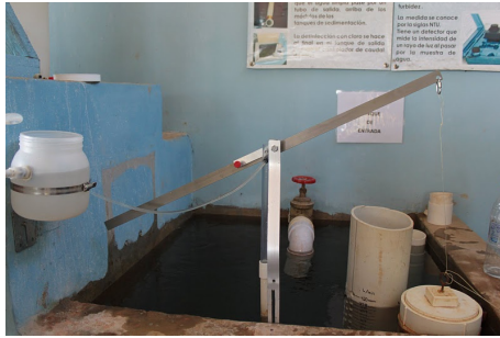
Figure 1: Chemical dose controller as installed at Agalteca. The dosing tube is too short in this installation resulting in a nonlinear response.
