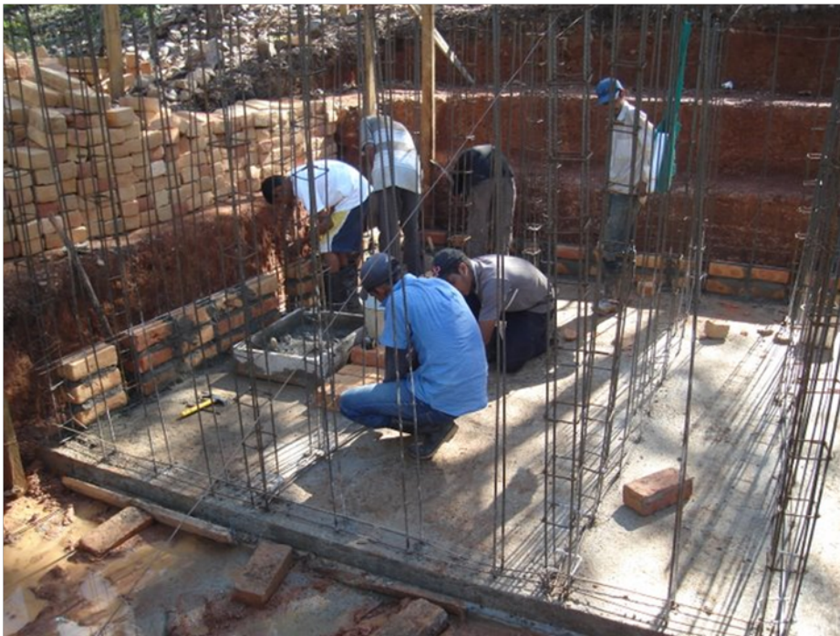
Figure 1: Poured slab reinforced foundation and bricks with both horizontal and vertical re-bar at the Agalteca water treatment plant.
