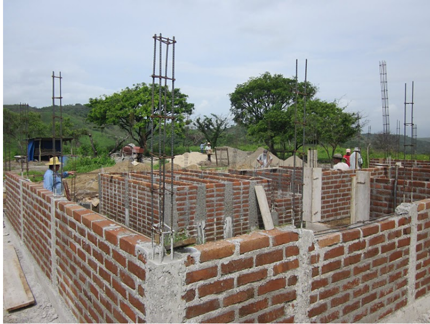
Figure 1: Bricks with Both Horizontal and Vertical rebar at the Alauca water treatment plant.
