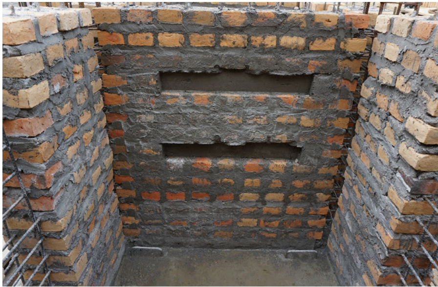
Figure 19: The rectangular channels with the depth of 5 cm and the height of 11 cm which will support the platform in Las Vegas, Honduras.
