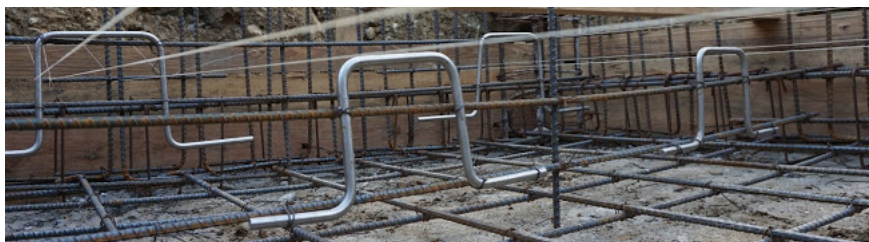
Figure 8: The stainless steel loop at the bottom of the tank in Las Vegas, Honduras.
