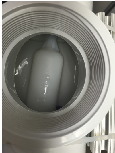
Figure 5: The aerial view of the custom made mini-float valve inside of the CHT.
