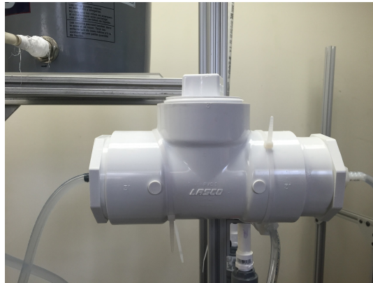
Figure 4: The spring 2015 CDC teams chlorine resistant CHT design housed by a 3 inch PVC tee. The design does not prevent stratification and is in a white tank that makes it harder for the operator to see inside.
