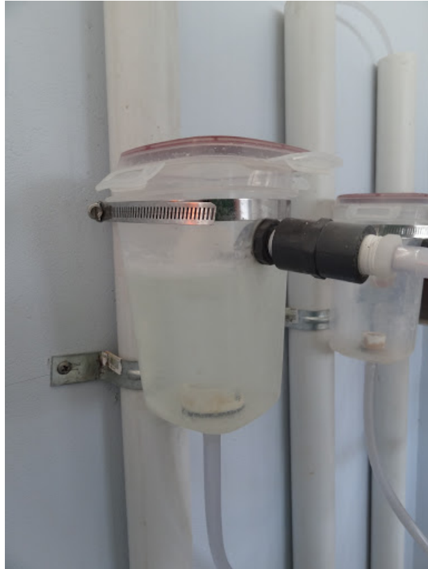
Figure 24: Photograph of a CHT used in Moroceli, Honduras which uses the first alternative connection between the mini adjustable PVC float valve with 3/8" parallel threaded inlet and the flexible tubing from the Chemical Stock Tanks. Unfortunately, the connection between the coupling and the float valve is not completely water tight.
