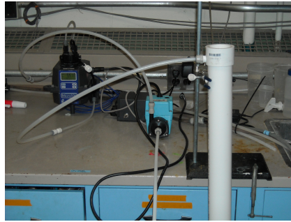
Figure 9: Close up of Pump Setup
