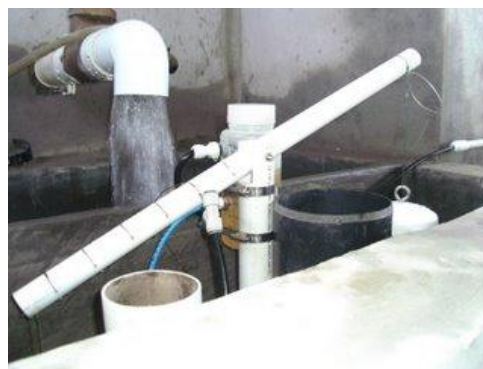
New chemical doser and linear flow orifice meter (LFOM) in the entrance tank
