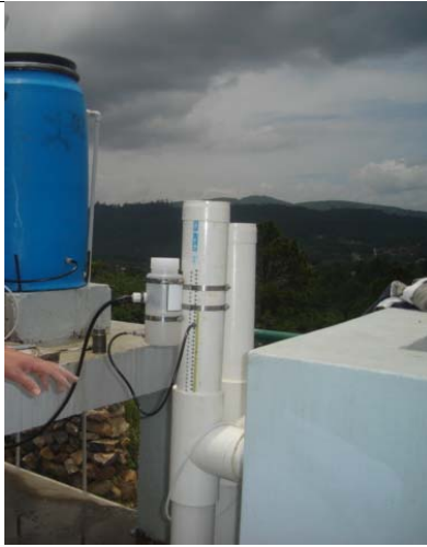
Figure 5. Alum flow controller installed in Ojojona, Honduras. The tank at the right is the entrance tank and the vertical pipe below the dosing tube is the rapid mix.
